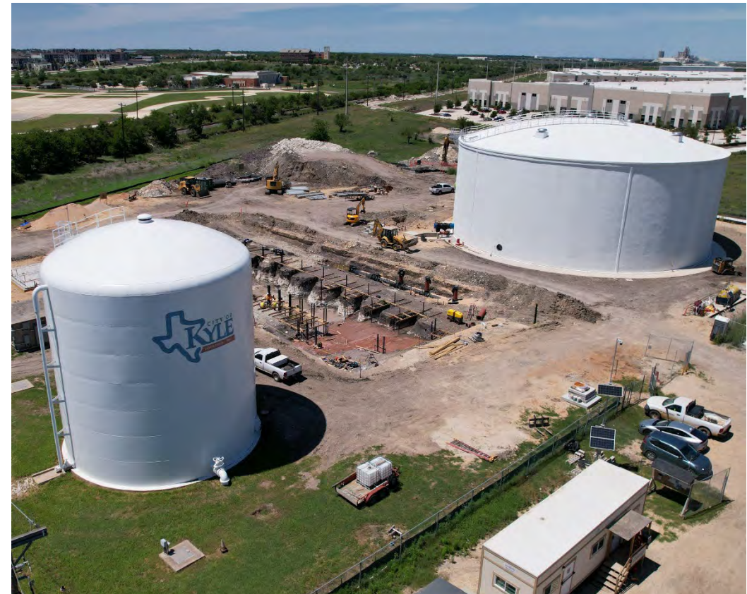
FM 1626 Take Point and Water Tanks
